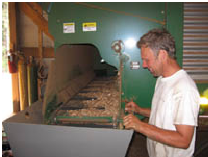
West End co-owner Dwayne Vanden Akker stands next to the fuel hopper for the new wood-fired boiler.
