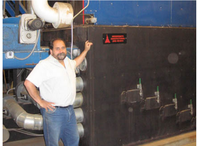
Rob Rizzo, Director of Renewable Energy Studies at MWCC stands next to the 8 MMBTU wood fired boiler that replaced an expensive electric heating and cooling system.
